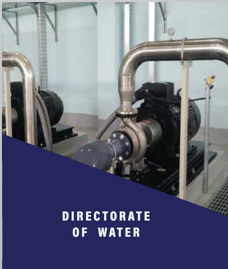
Sulayyil Reverse Osmosis plant 10,000 m3/d Capacity
